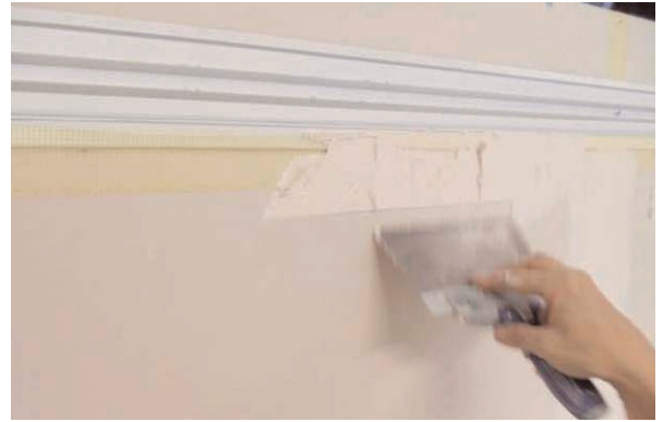
2) Plaster or other compound is blended over the lower portion of the Rail and feathered down the wall, eliminating minor inconsistencies in wall straightness.
