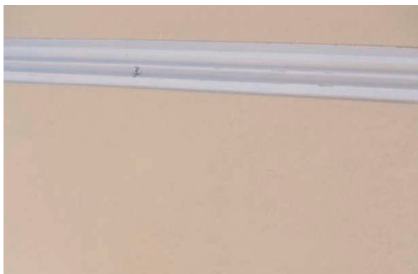
3) The wall is textured and finished, leaving a perfectly straight channel, ready to receive the fixture's reflector assembly.
